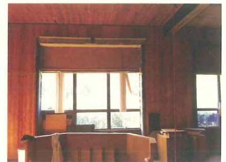
The interior of the firehouse after the ceiling and walls have been stripped.
