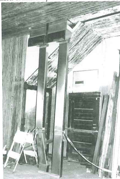
New 21 st century ducts for geothermal HVAC in the 19 th century building.
