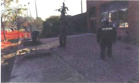
McAdam Landscaping staff installed the vintage paving blocks (Photo by Frank Lipo)
